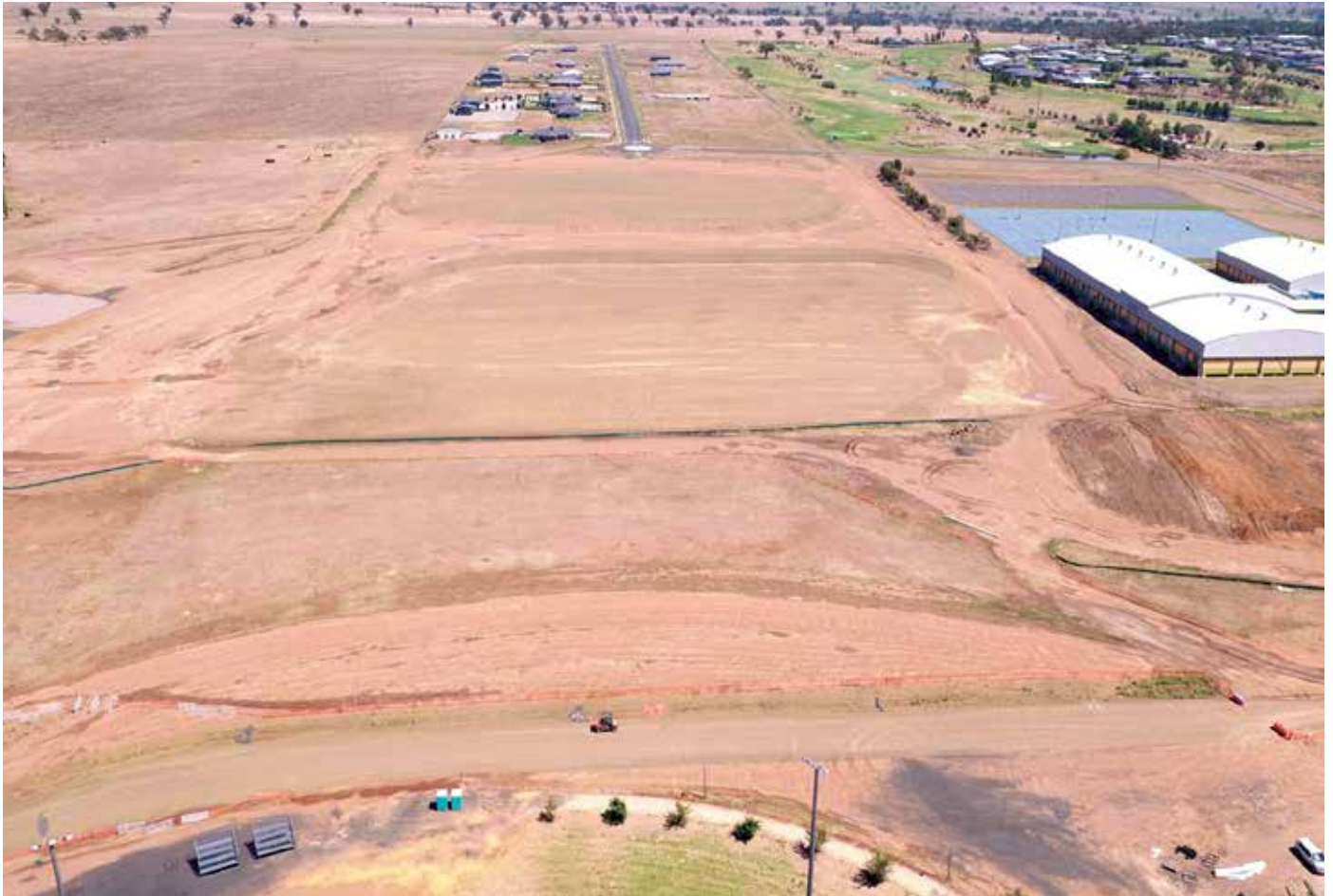
An image captured from a drone looking towards Rodeo Drive and showing the earthworks for the new athletics and cycling facilities behind the Sports Dome.
