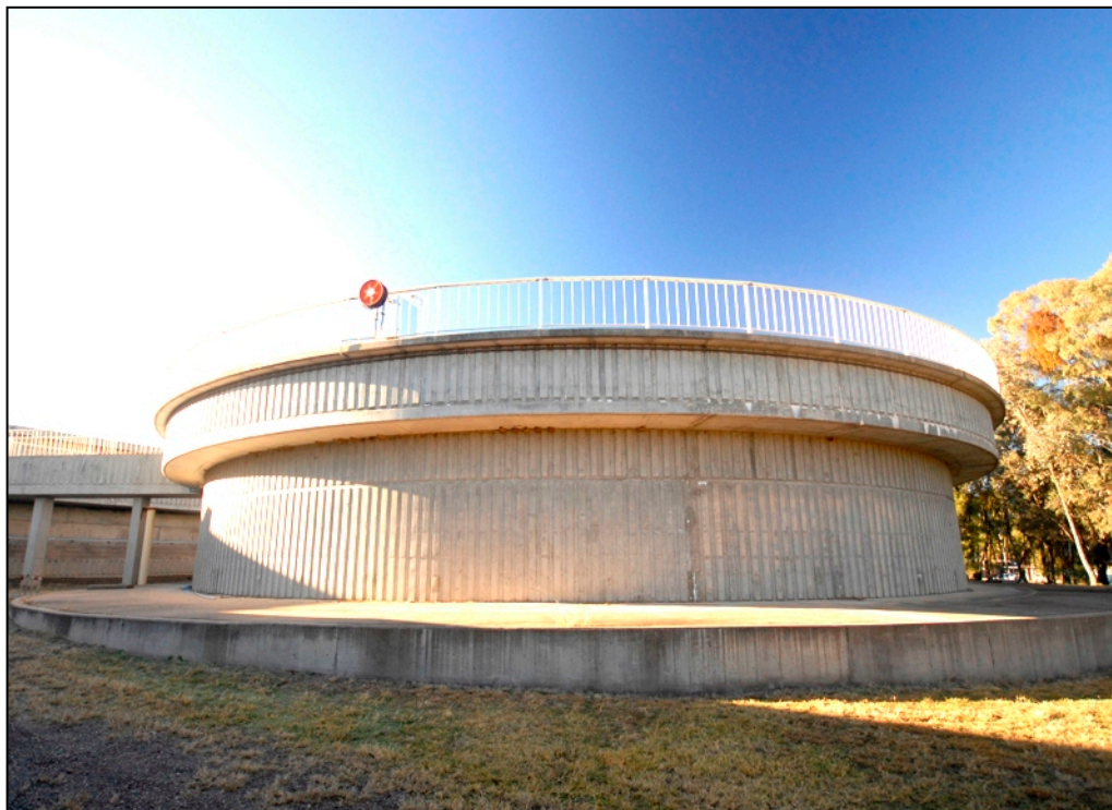
Clarifier tank at Calala Water Treatment Plant
