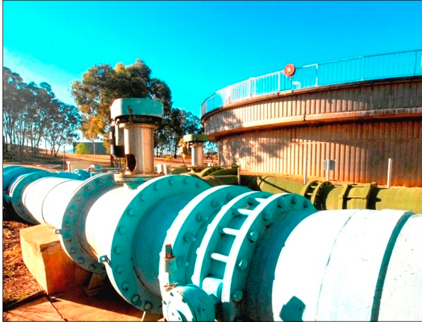
The inflow pipes at Calala Water Treatment Plant (WTP)
